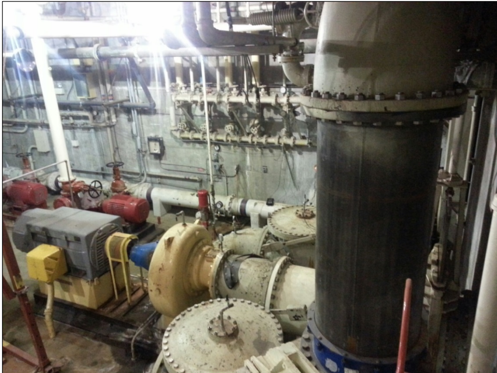
Figure 4: Process Water (3W) Pump Station
