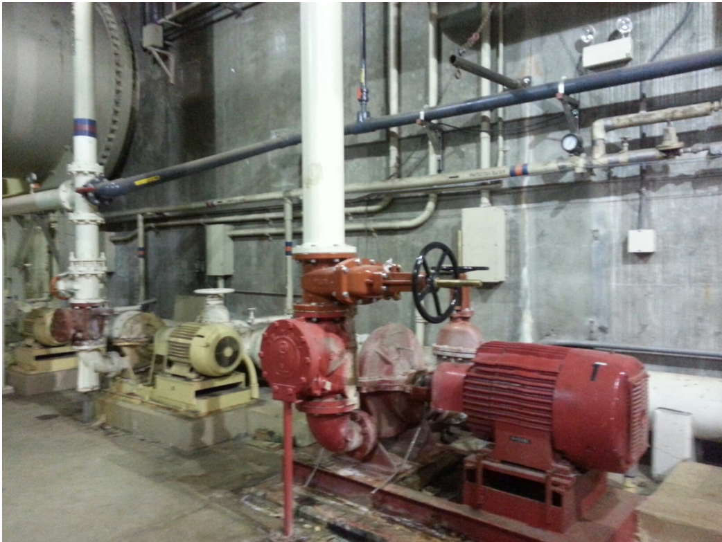
Figure 3: Fire Protection Water Pumps
