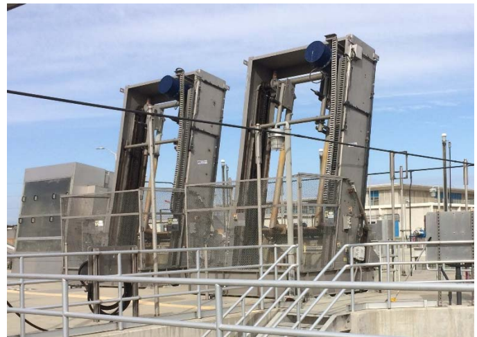
Figure 4: Headworks 1 Bar Screens
