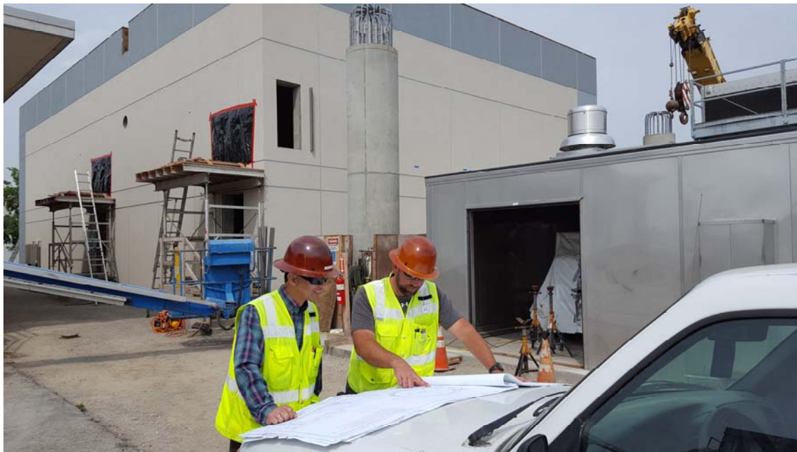
Figure 1 – Assoc. Engineer Rene Apelo and Sr. Inspector Allan Morgenroth Collaborate at the Digester Gas Compressor Upgrades Project
