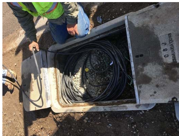
Figure 4: Fiber coiled in new pull box
