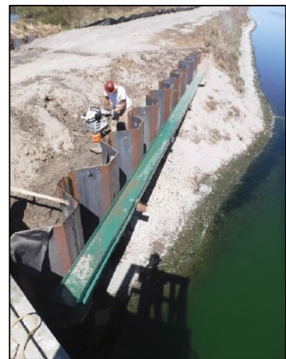
Levee was reinforced with sheet piles and horizontal whalers to prevent erosion and shifting.
