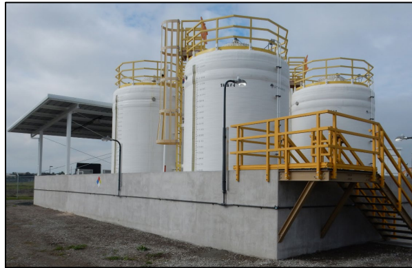
Iron Salt Feed Station.
