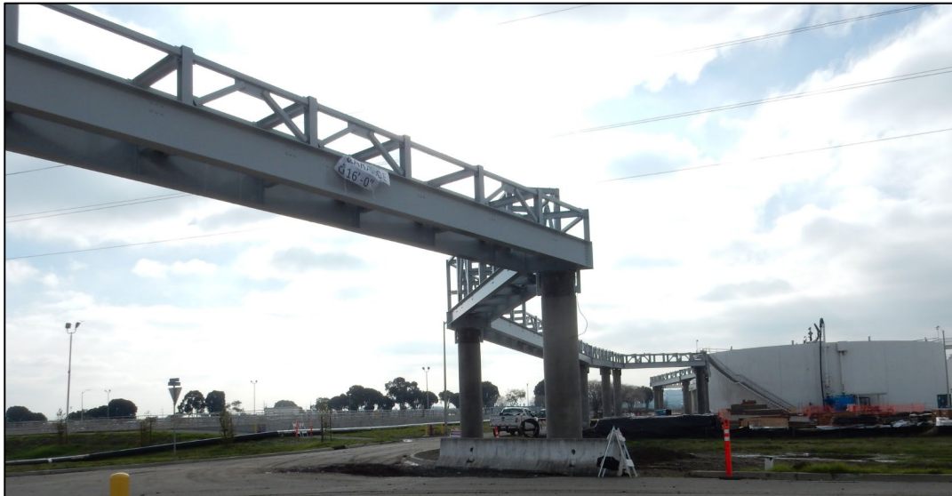
New permanent above-ground piping racks: “The Monorail.”
