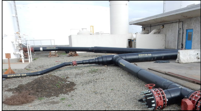
Temporary digester gas above-ground (on-ground) piping
