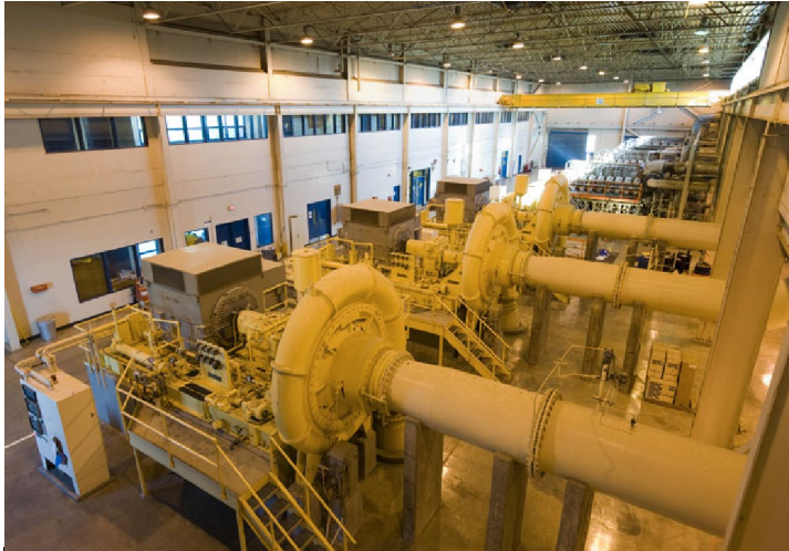
Process Air Blowers, PAB-1 thru PAB-3.
