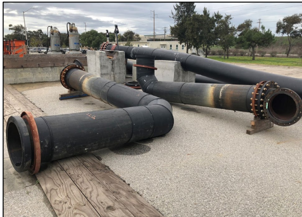
Sections of 36-inch HDPE pipe, installed and used as a temporary piping system while the 78" PE line was out of service for repair.
