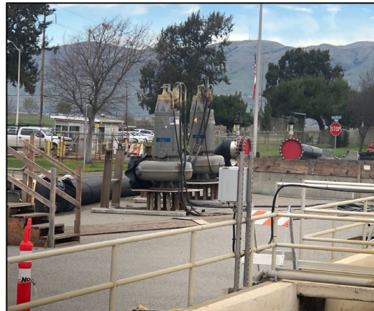
Two of the pumps utilized in the temporary piping system while the 78" PE line was out of service for repair.
