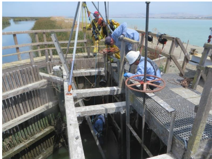
Figure 26. City personnel replacing the slotted fish screens to allow for outflow through the southern structure
