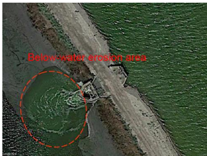
Figure 23. Google Earth satellite imagery details the erosion on the outboard side of the southern hydraulic structure
