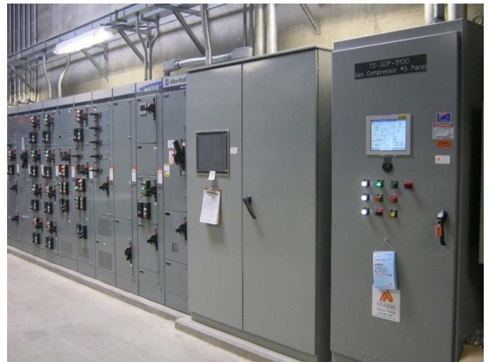
Figure 7: Digester Gas Compressor Electrical Room Control Panels
