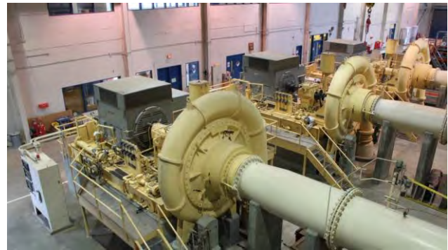
Electric Blowers in Building 40
