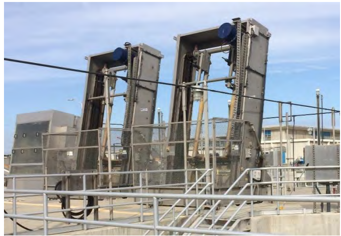
Headworks 1 Bar Screens
