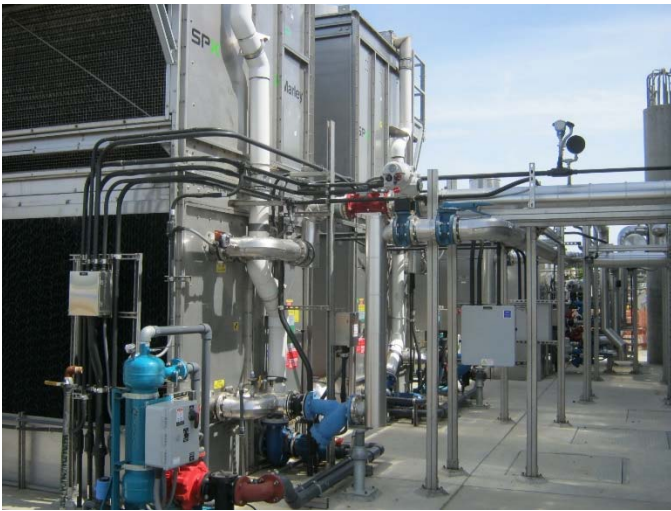
Figure 6: Digester Gas Compressor Cooling System
