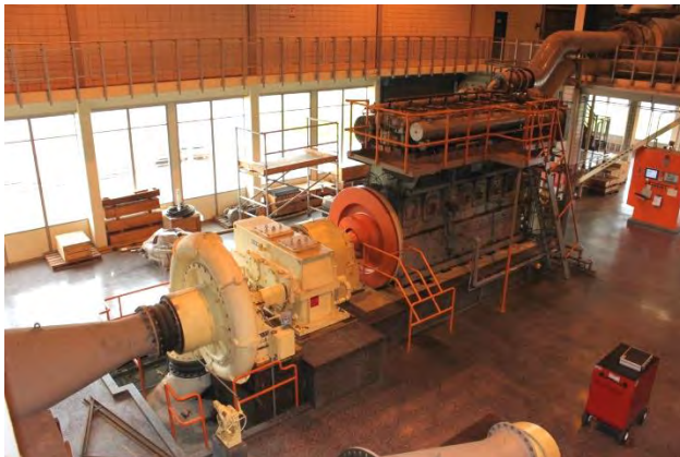
Engine-driven Blower in Secondary Blower Building
