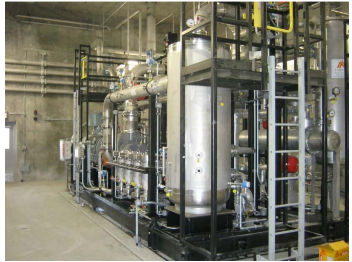
Figure 5: Digester Gas Compressor Skid
