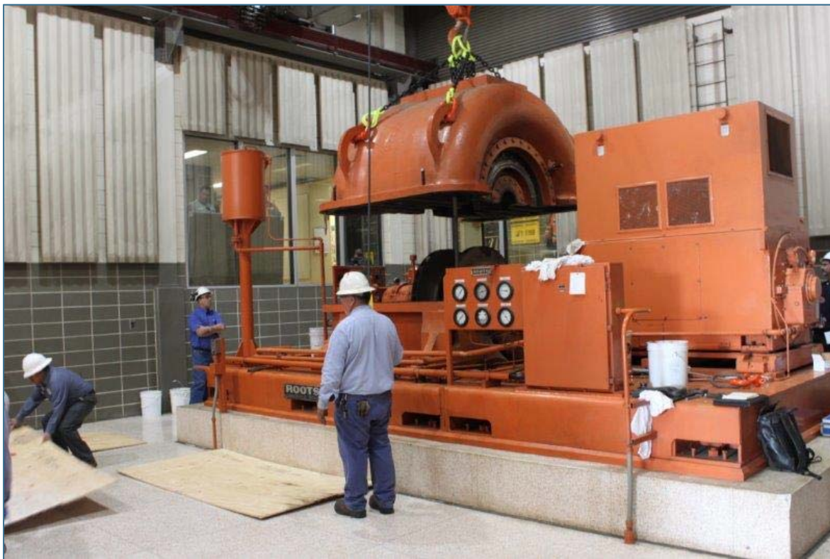
Figure 2: Existing Engine Blower
