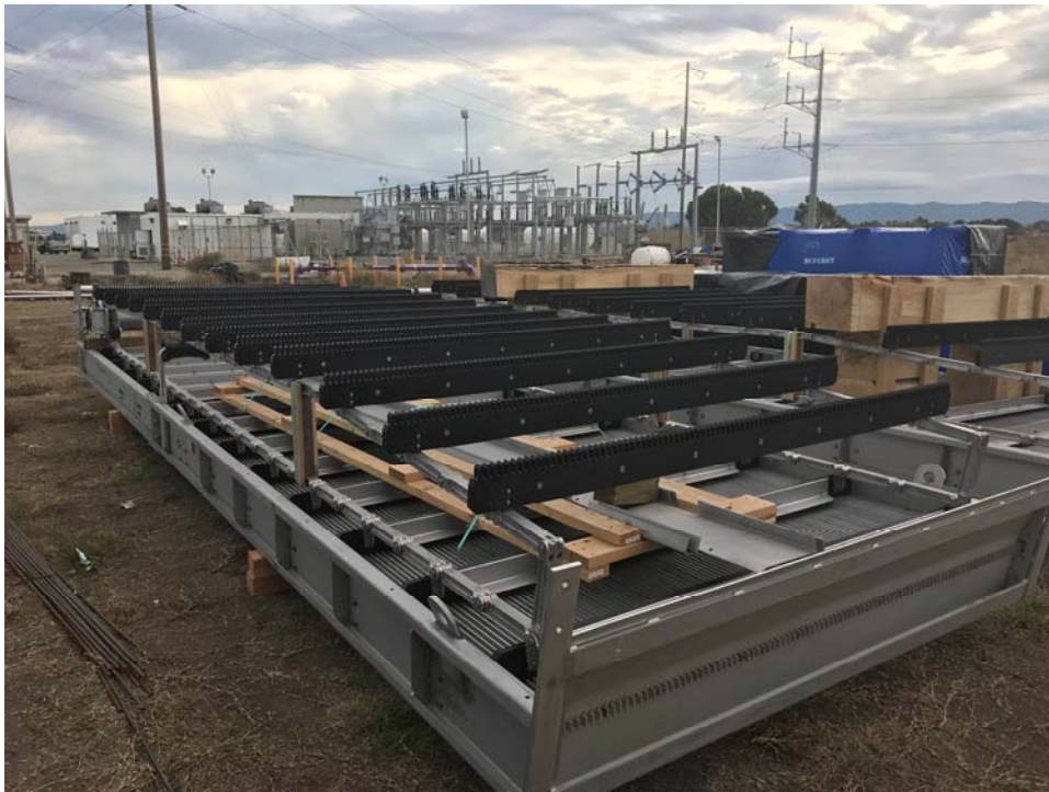
Figure 5: New Bar Screens
