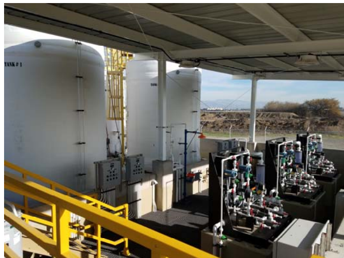
Figure 3: Ferric Chloride Station
