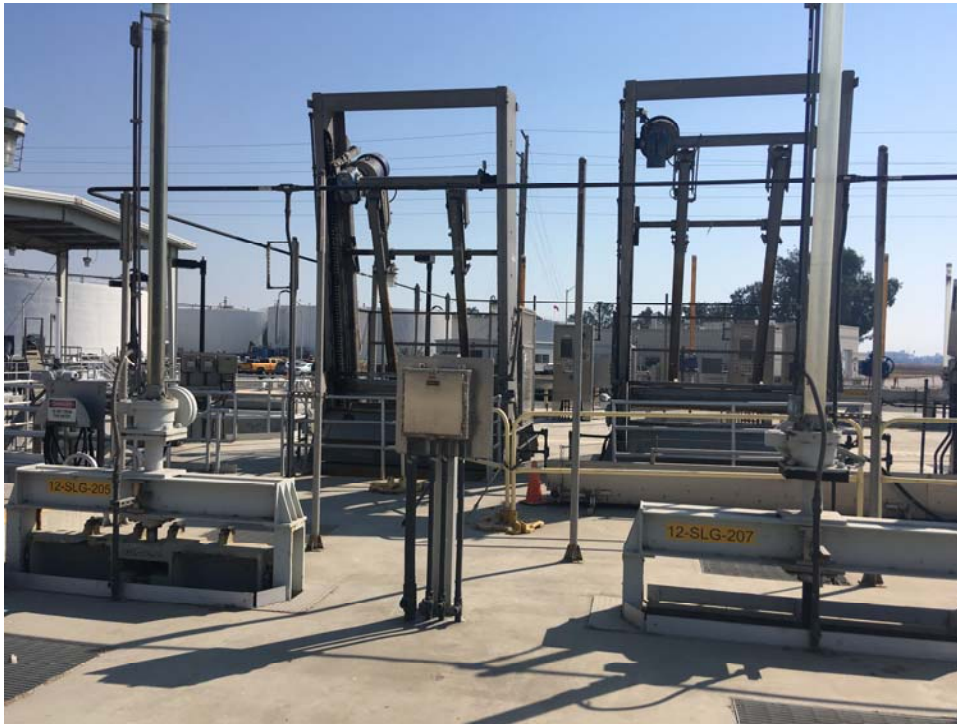
Figure 4: Current Bar Screens
