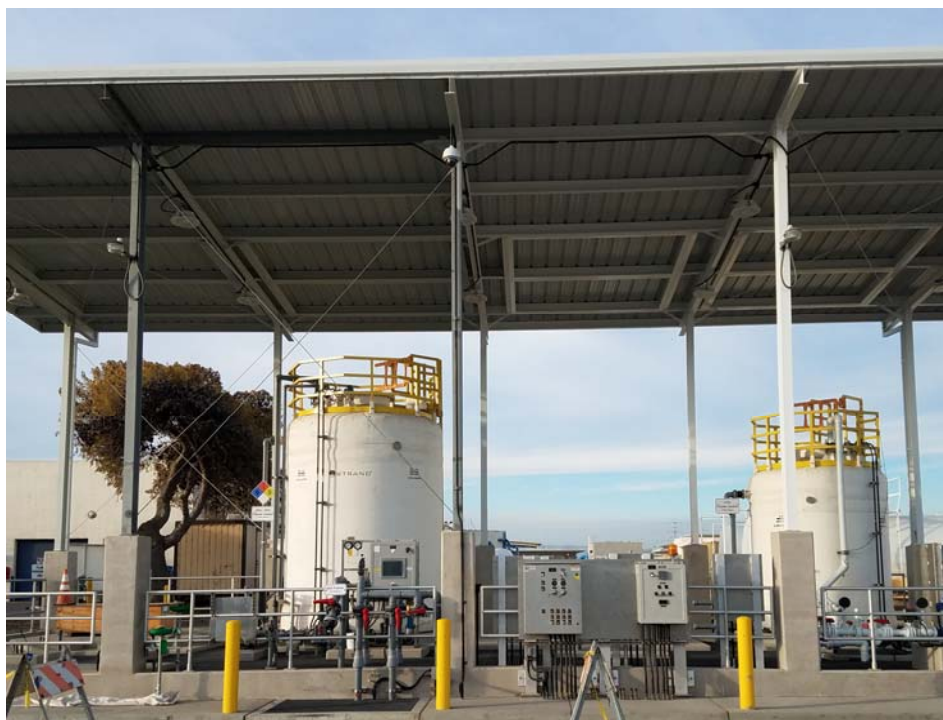
Figure 4: Polymer Feed Station
