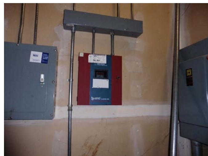
Figure 4: Fire Control and Communicator in CL/SO2 Building
