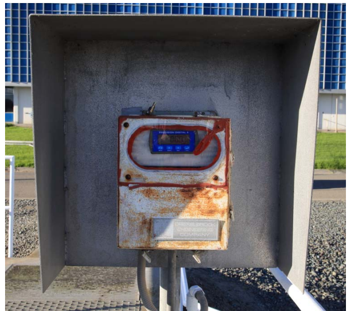
Figure 7: Existing Effluent Flow Meter at the Secondary Clarifier
