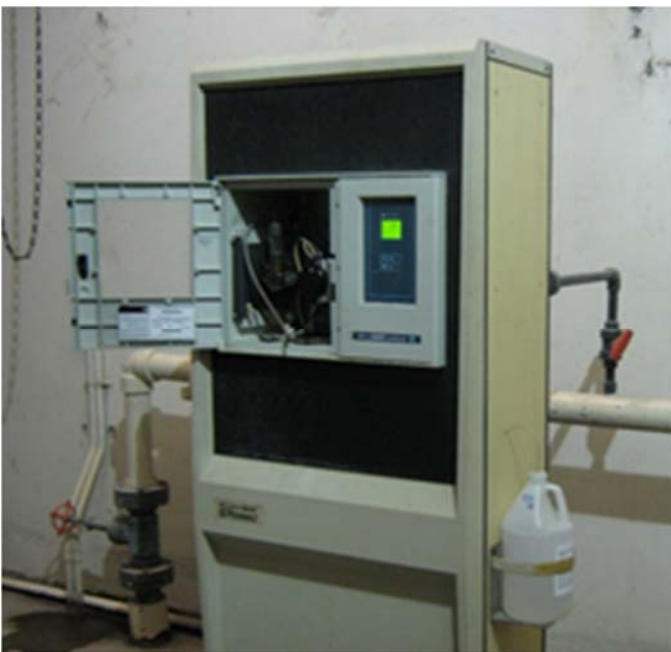
Figure 6: Filter Building Chlorine Analyzer
