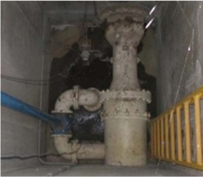
Figure 4: RAS Flow Meter
