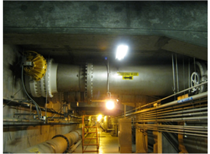
Figure 5: Secondary Settled Sewage Influent Flow Meter
