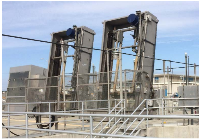
Headworks 1 Bar Screens
