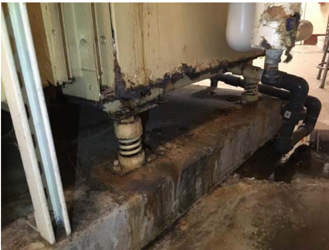
Figure 4: Heavily Corroded Air Handler Unit
