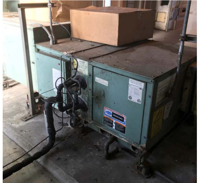
Figure 3: Aging Air Handler Unit
