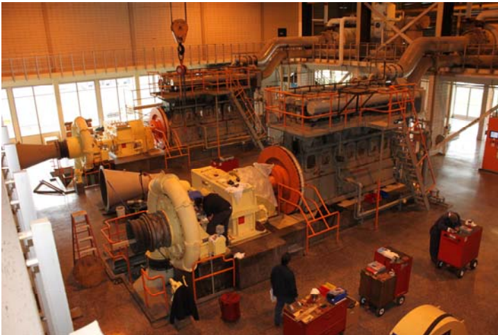
Figure 2: B-2 Blower that will be converted to an electric motor under the project scope
