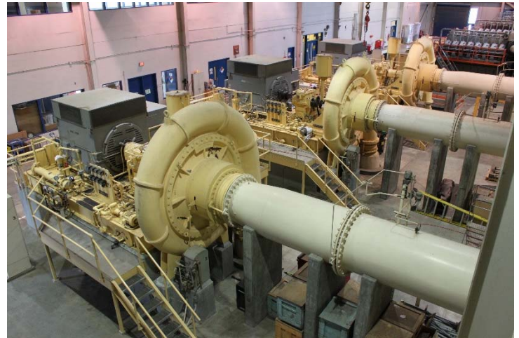
Figure 3: Blower Generator Building 4,000 hp Aeration Blowers
