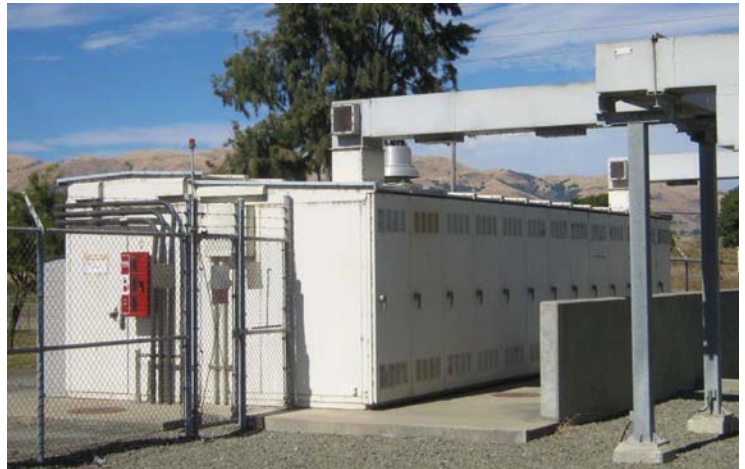
Figure 3: Exterior of Existing M4 (5kV) Switchgear Enclosure
