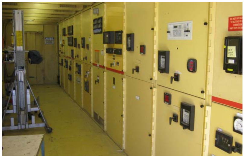
Figure 4: Interior of Existing M4 (5kV) Switchgear Enclosure
