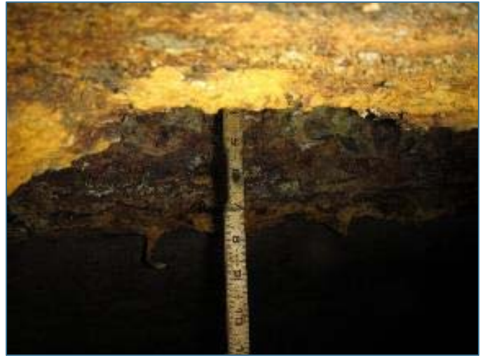
Figure 4: Crown corrosion pocket on 96-inch SES Pipeline
