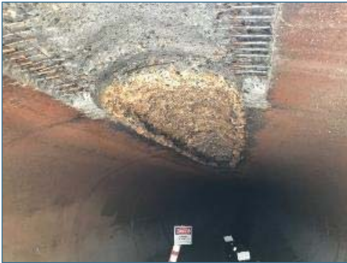
Figure 5: Crown corrosion of 87-inch SES Pipeline
