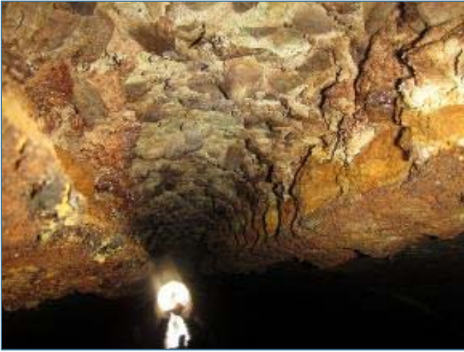
Figure 3: Rebar degradation on 96-inch SES Pipeline
