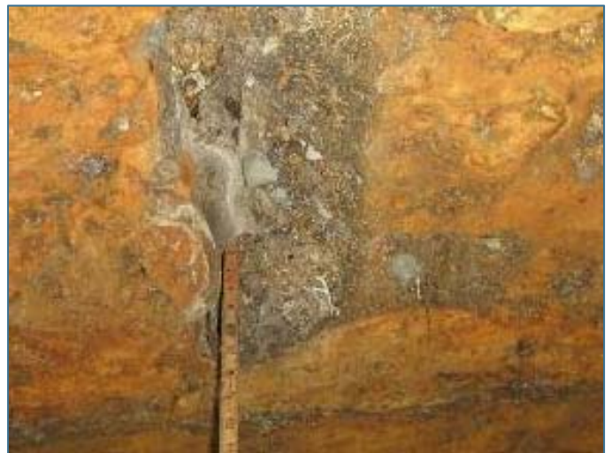
Figure 6: Crown corrosion pocket of 87-inch SES Pipeline
