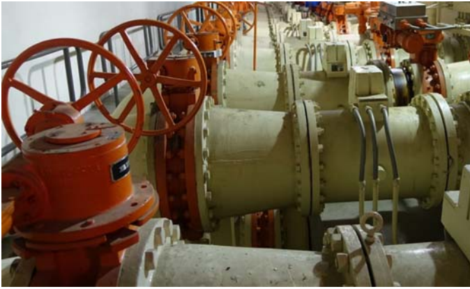
Figure 3: RAS Pipeline Gallery in Tertiary Blower Building
