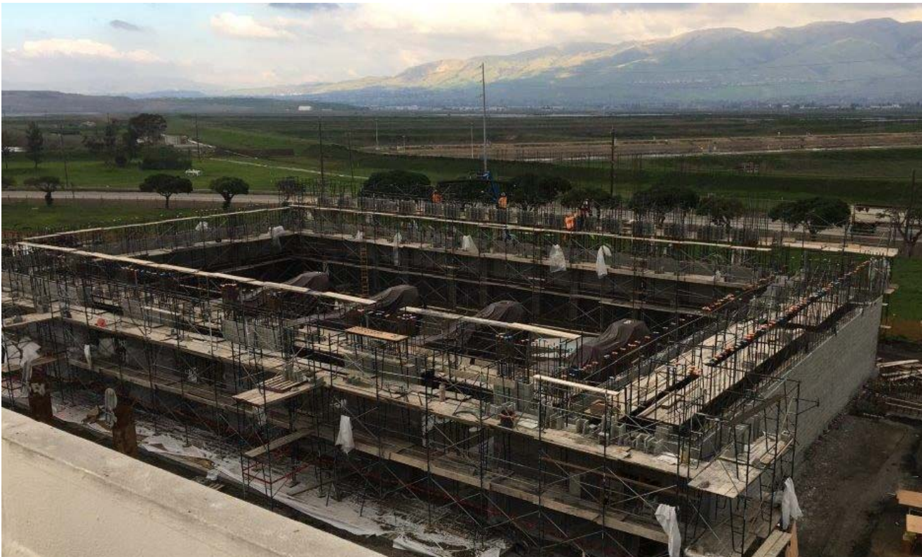
Figure 3: Main Cogeneration Building
