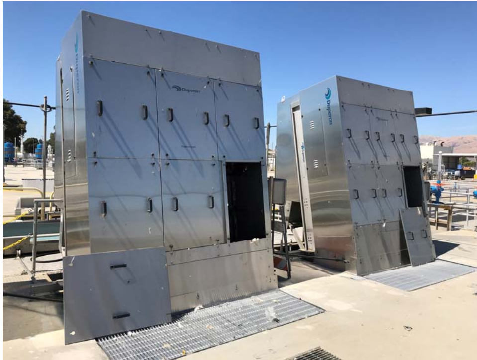
Figure 6: New multi-rake bar screens at Headworks 2, installed under the recently completed Headworks Critical Improvements Project. Similar screens are planned to be installed at Headworks 3.
