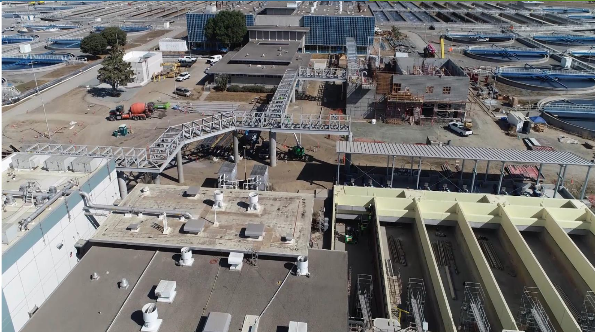
Digester Upgrades: Aerial overview of Piperack, DAFTS 1-6, the new thickened sludge pump canopy and new sludge screen building
