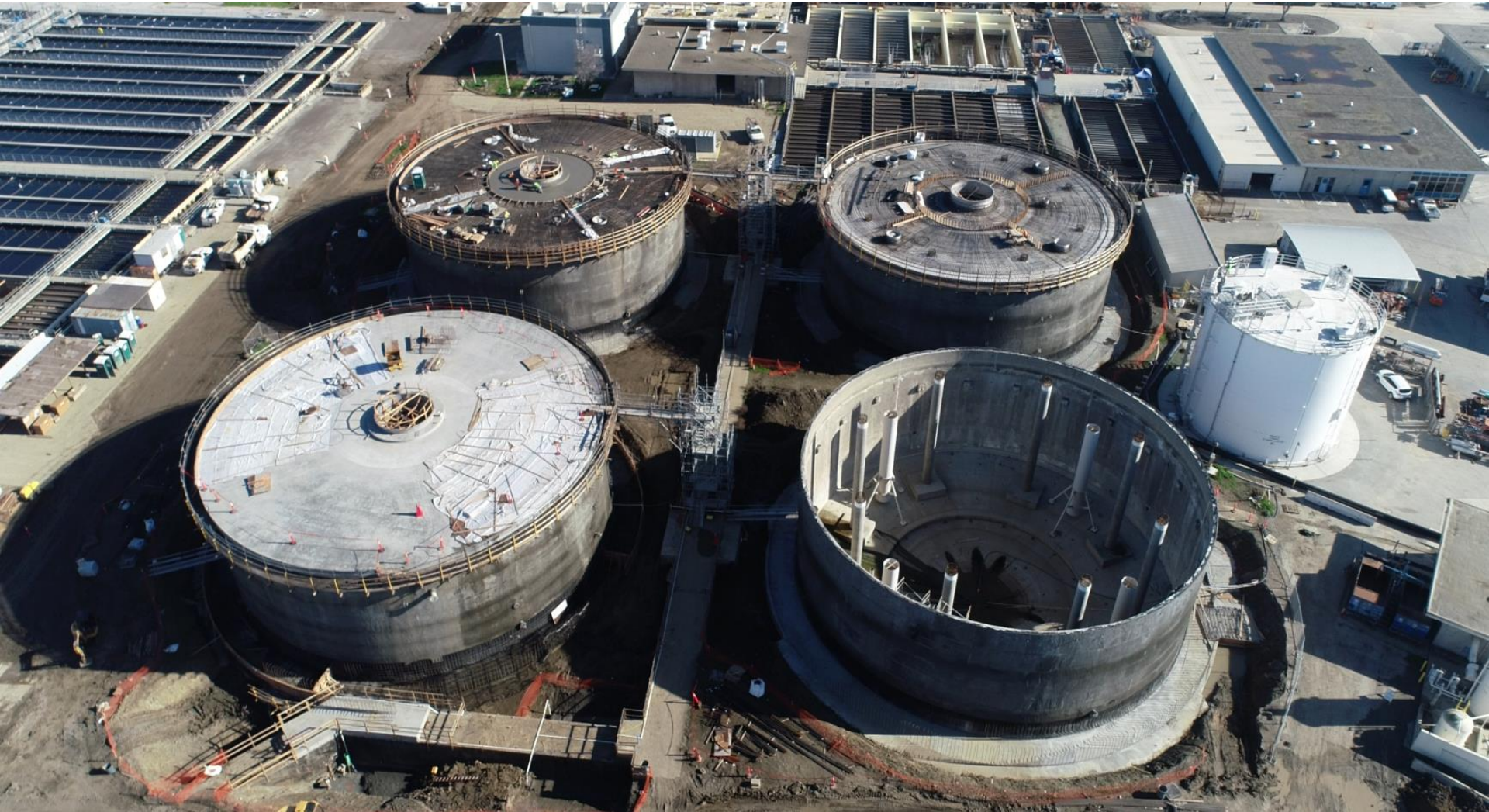
Digester Upgrades: Formwork for the seismic ring and concrete pour roofs for Digester 5-8.
