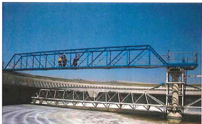
Clarifier Interior and Mechanism
