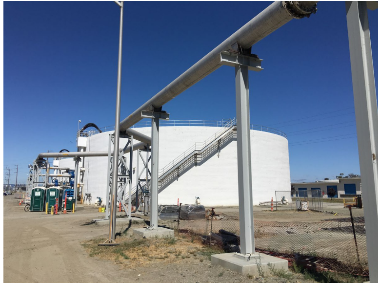
Figure 1: Digester 16 elevated gas line.
