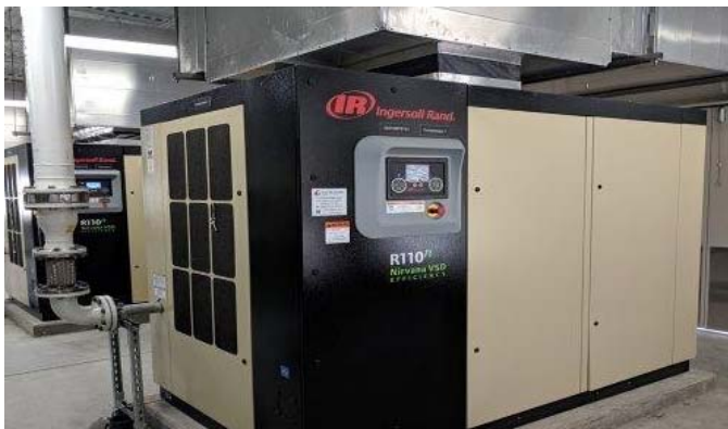
Figure 7: New Air Compressors
