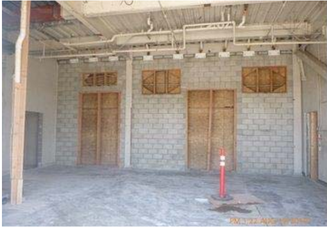
Figure 4: New VFD room in Building 40
