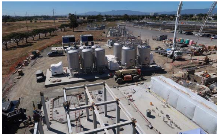
Figure 3: Bottom left: Pipe support structure under construction. Middle: Hydrogen sulfide and siloxane removal equipment. Middle right: Electrical ductbank concrete pour.
