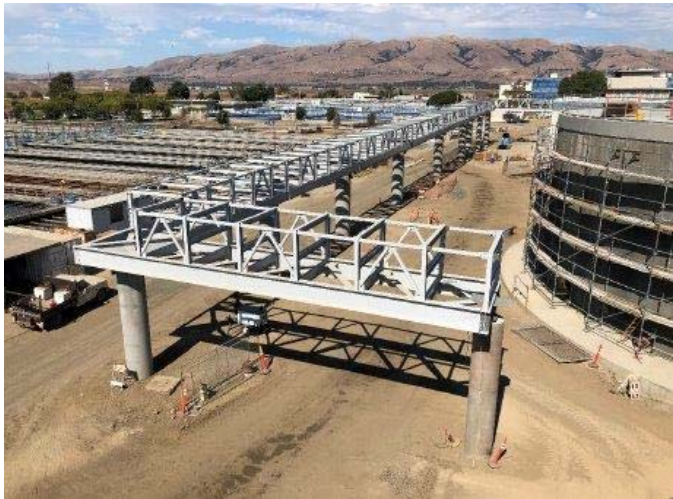
Figure 2: Pipe rack system and Digester 6
