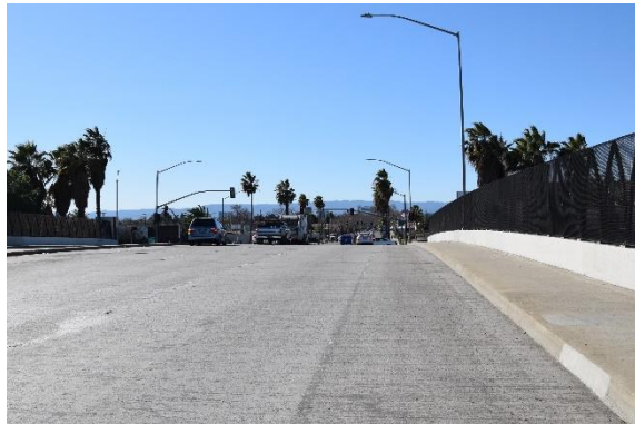
Narrow Sidewalks on Freeway Overpasses
