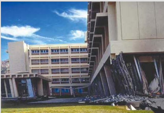
Damage to hospital in 1971 San Fernando Earthquake
