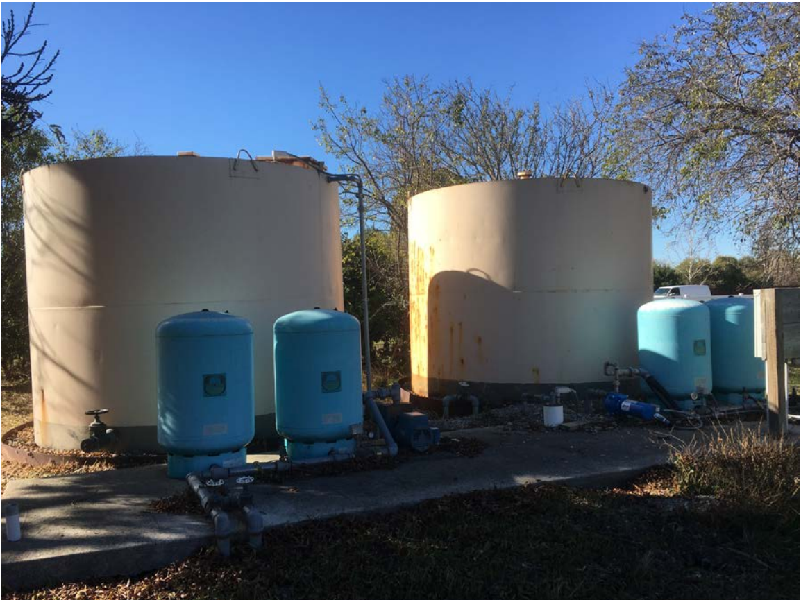
Photograph 4 - Water tanks, pressure tanks and electric motors on Property
