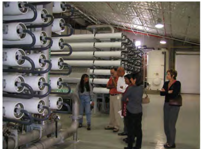
Figure 1: Reverse osmosis plant at Alameda County Water District works to remove excess minerals.
