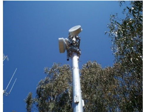
ECOMM Antennae at Eagle Rock
