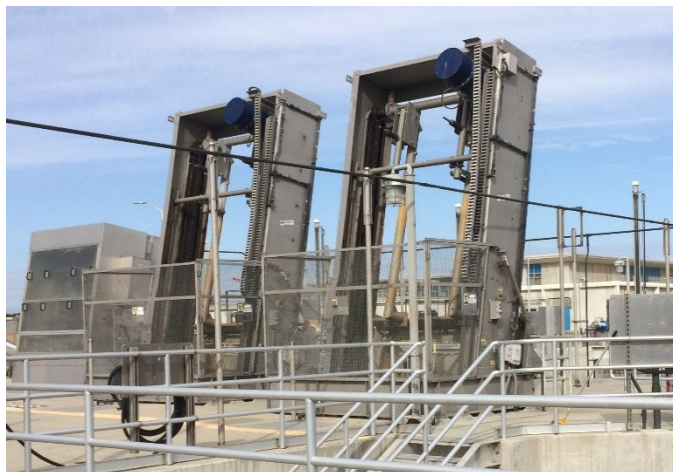
Headworks #1 Bar Screens
