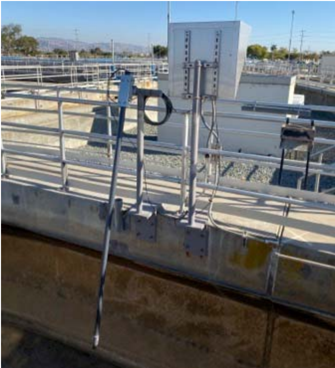
Figure 7: New Total Suspended Solids Sensor and Transmitter at the Secondary Mix Liquor Channel
