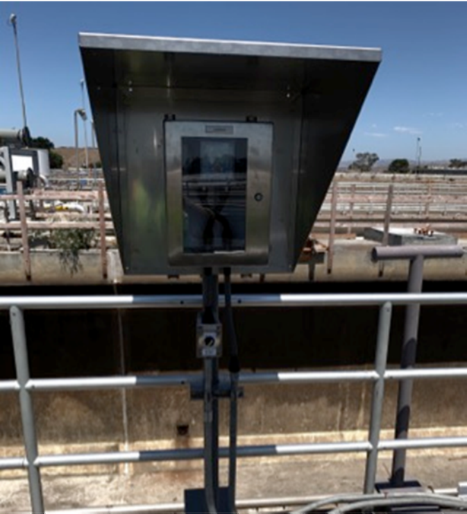
Figure 8: New Dissolved Oxygen Transmitter at the Secondary Aeration Basins
