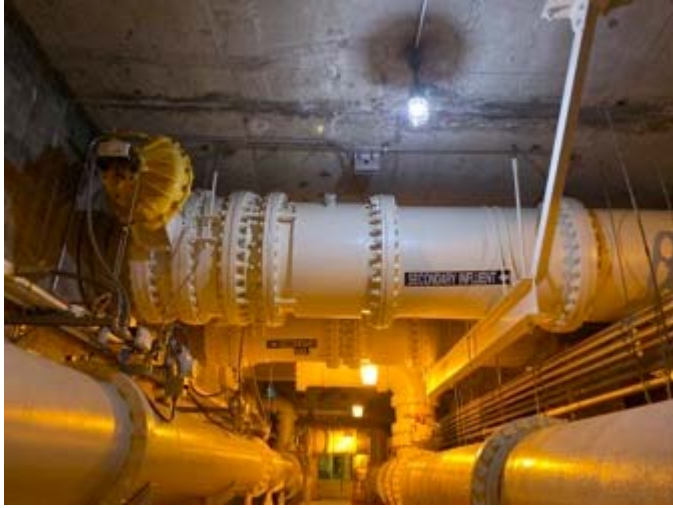
Figure 6: New Secondary Settled Sewage Influent Magnetic Flow Meter
