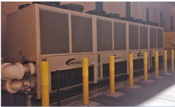
* Civic Auditorium Air Conditioning
