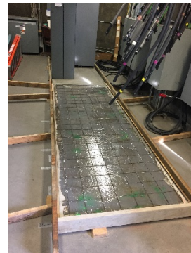
*PAC Electrical System Upgrade
