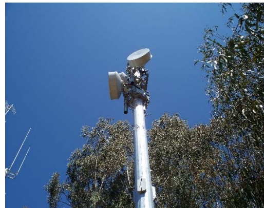
ECOMM Antennae at Eagle Rock
