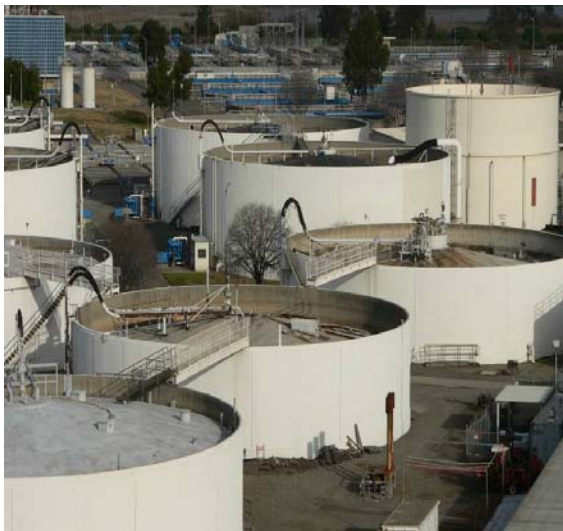
Existing Digester Facilities
