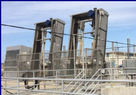
Headworks 1 Bar Screens
