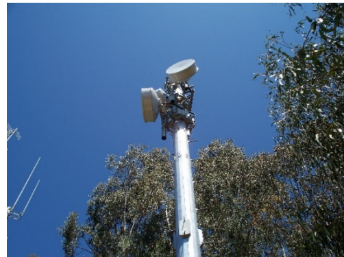
Emergency Communications Microwave Antennae at Eagle Rock
