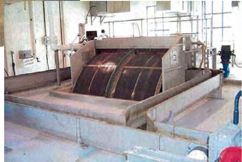
Figure D-2 DRUM SCREENS FOR INFLUENT FINE SCREENING SAN JOSÉ/SANTA CLARA WPCP MASTER PLAN CITY OF SAN JOSÉ
