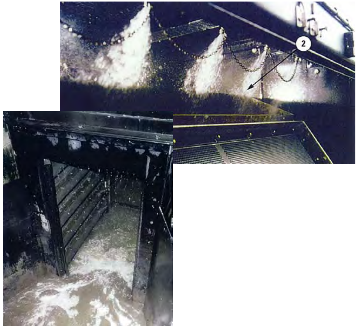
Figure D-1 BAND SCREENS FOR INFLUENT FINE SCREENING SAN JOSÉ/SANTA CLARA WPCP MASTER PLAN CITY OF SAN JOSÉ
