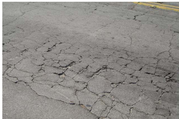
City Street in "poor" pavement condition
