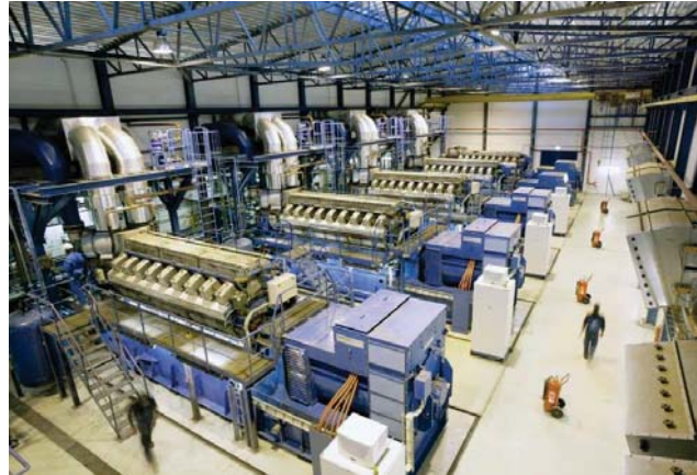
Internal combustion engines similar to the ones planned for the Cogeneration Facility
