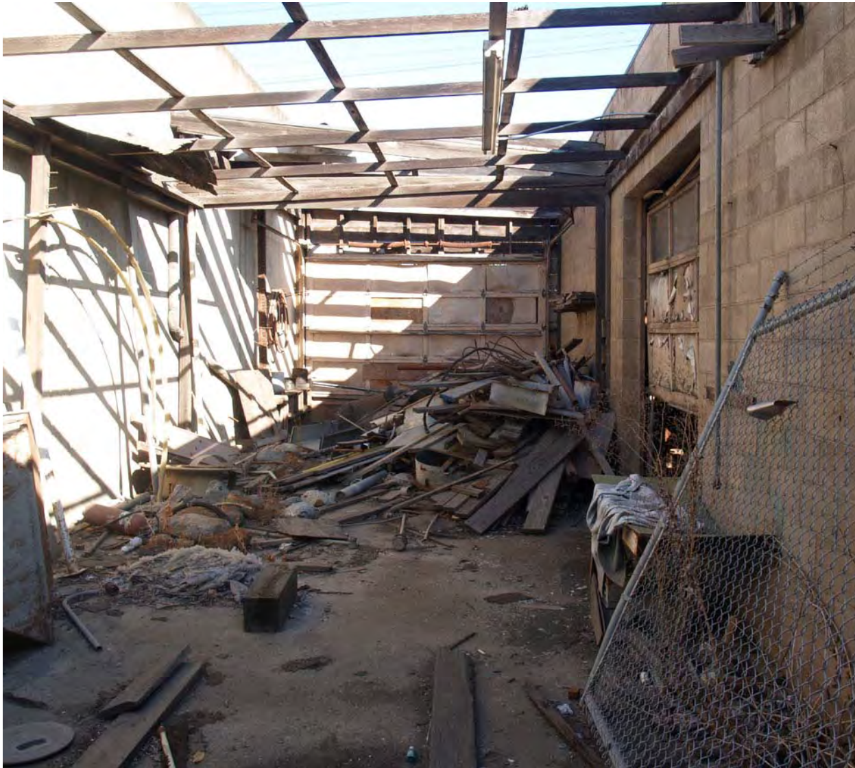
Space between Westinghouse building and ancillary building to rear, viewed Facing northwest
