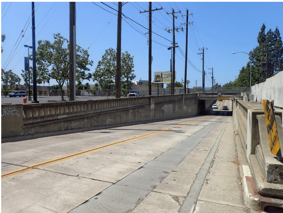
Entry to underpass from east near North Montgomery Street, viewed facing southwest.
