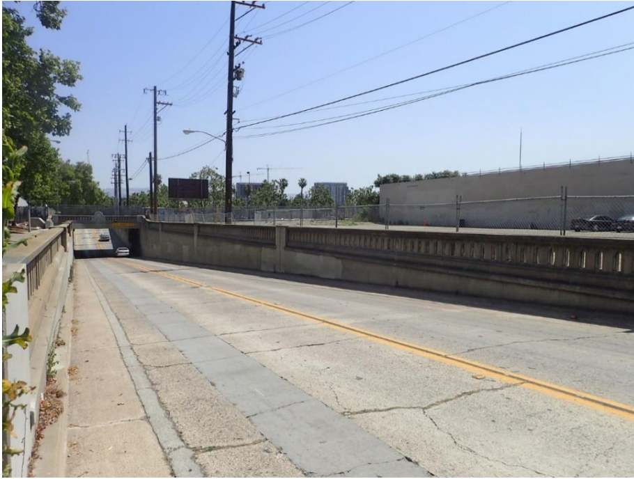
Bridge and underpass with subject project site to the right, viewed facing east.
