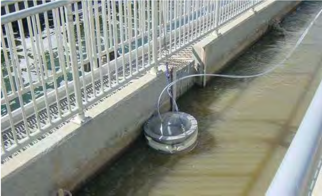
Figure F-1 Flux chamber used to collect air sample from an isolated headspace
