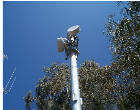
ECOMM Antennae at Eagle Rock
