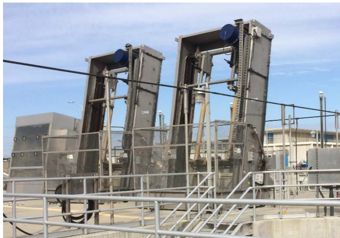
Headworks #1 Bar Screens
