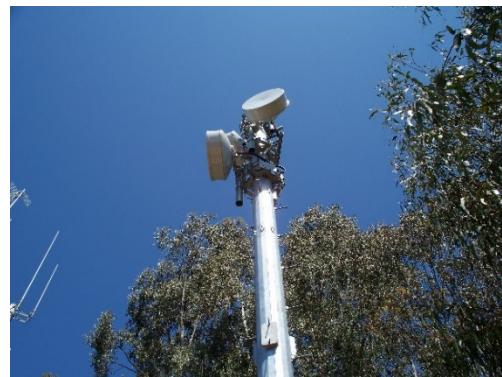
Emergency Communications Microwave Antennae at Eagle Rock
