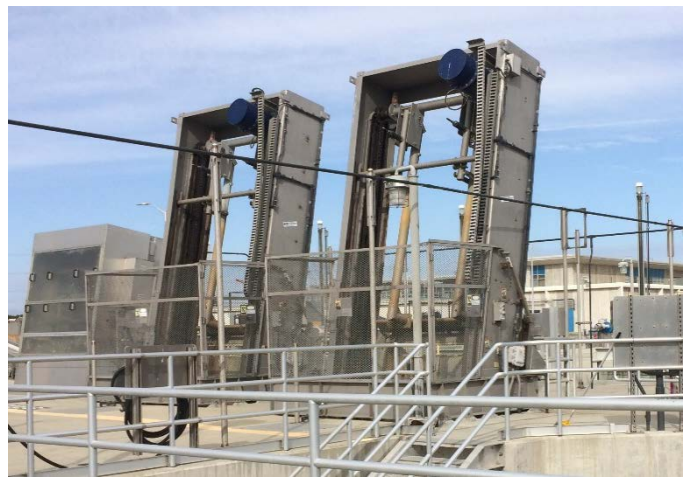
Headworks 1 Bar Screens
