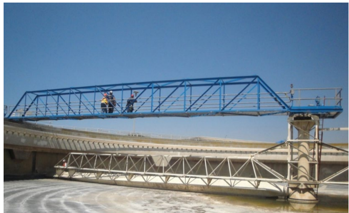
Clarifier Interior and Mechanism
