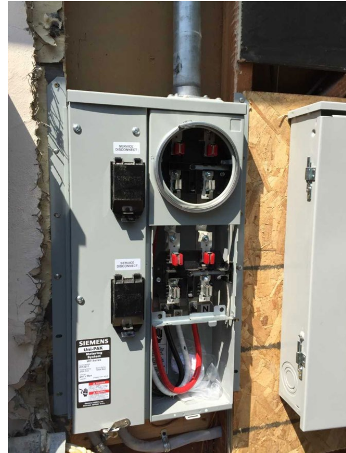
New Electrical Service Panel
