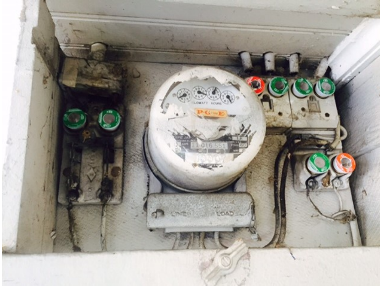
Old Electrical Service Panel
