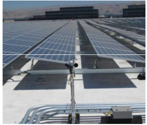
Solar installation at San Jose Mineta International Airport (SJC)
