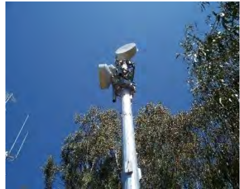
ECOMM Antennae at Eagle Rock
