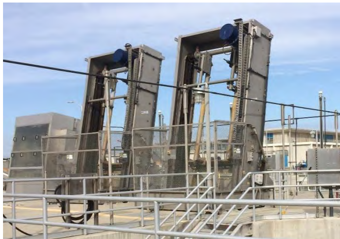
Headworks #1 Bar Screens
