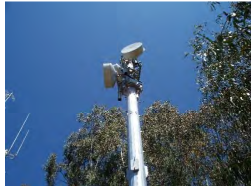
Emergency Communications Microwave Antennae at Eagle Rock
