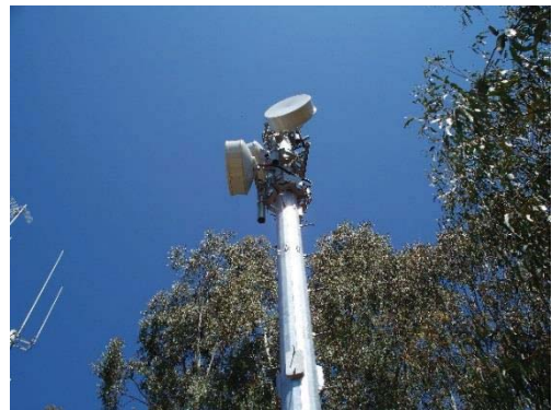
Emergency Communications Microwave Antennae at Eagle Rock
