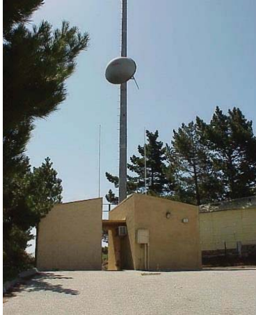
Cadwallader Reservoir Radio Tower
