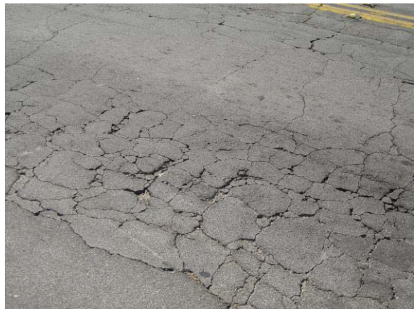
City Street in "poor" pavement condition
