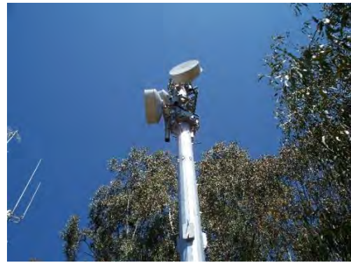
Emergency Communications Microwave Antennae at Eagle Rock
