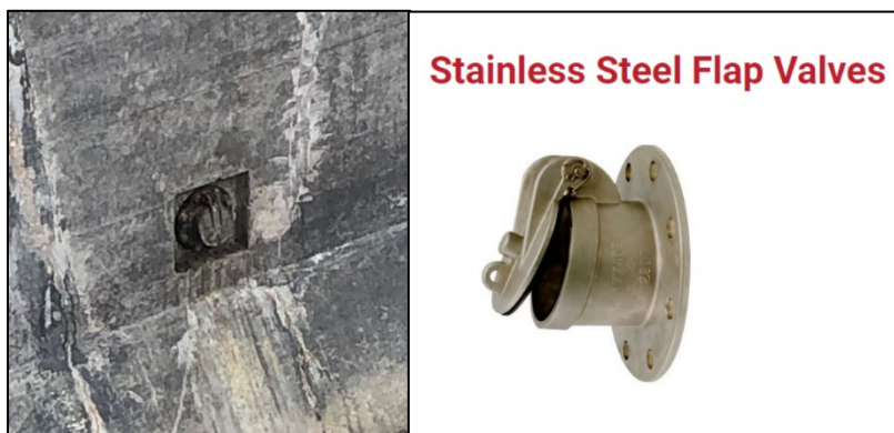
FIGURE 43 ALL FLAP VALVES GROUNDWATER PRESSURE RELIEF VALVES LIKE THE ONE IN BNR-1 (LEFT) WILL BE REPLACED WITH NEW STAINLESS STEEL VALVES (RIGHT)
