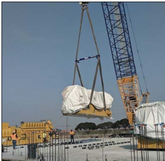
FIGURE 31 A 330-TON CRANE PLACED EACH OF THE FOUR COGENERATION ENGINES ON ITS BASE
