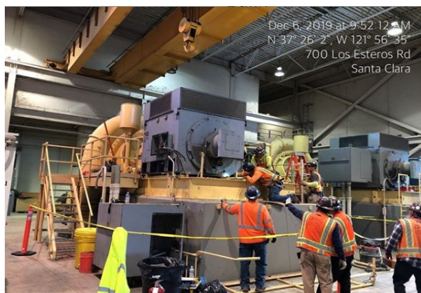
FIGURE 32 BLOWER IMPROVEMENTS PROJECT PREPARING TO INSTALL A NEW ELECTRIC MOTOR TO IMPROVE THE AERATION SYSTEMS’ RELIABILITY
