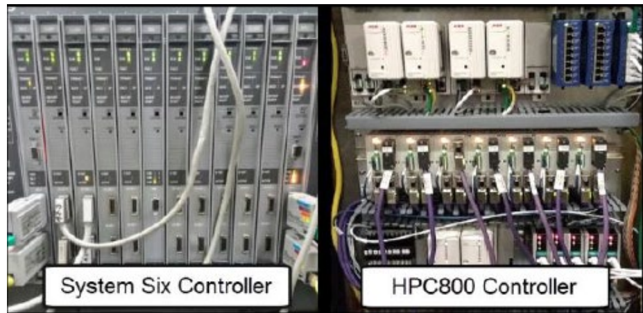
FIGURE 50 THE DCS WILL BE UPGRADE FROM SYSTEM SIX (LEFT) TO NEW HARMONY (RIGHT) CONTROLLERS
