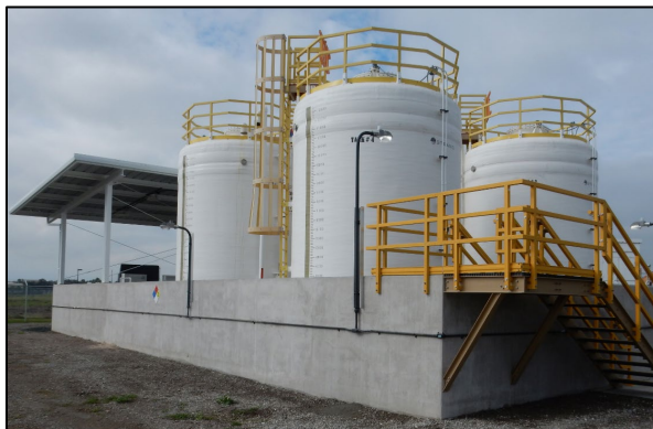
FIGURE 34 IRON SALT FEED STATION
