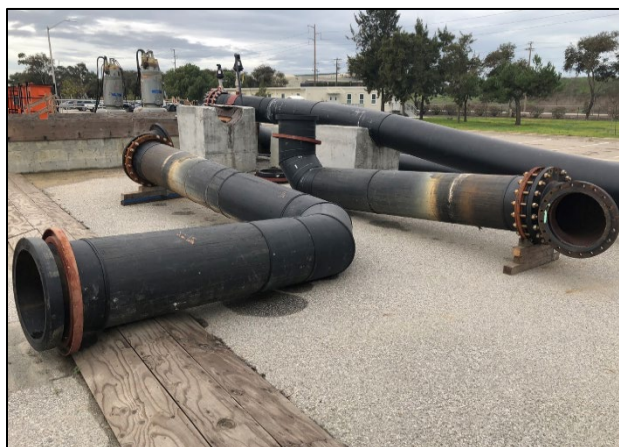
FIGURE 37 SECTIONS OF 36-INCH HDPE PIPE, USED AS A TEMPORARY PIPING SYSTEM IN 2018 THAT WILL BE USED AGAIN FOR THE SES REHABILITATION PROJECT
