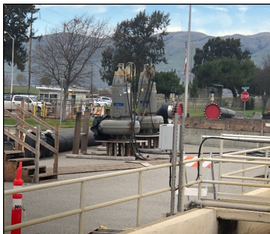
FIGURE 38 TWO OF THE PUMPS UTILIZED IN THE TEMPORARY PIPING SYSTEM THAT WAS USED IN 2018 AND WILL BE USED AGAIN FOR THE SES REHABILITATION PROJECT.
