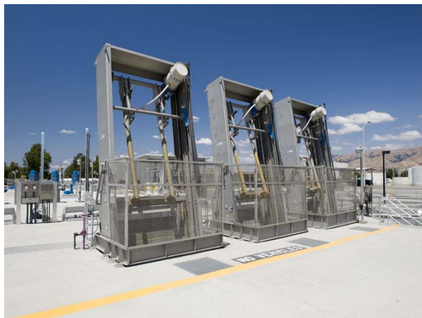
Headworks Bar Screens
