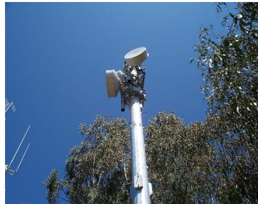
ECOMM Antennae at Eagle Rock
